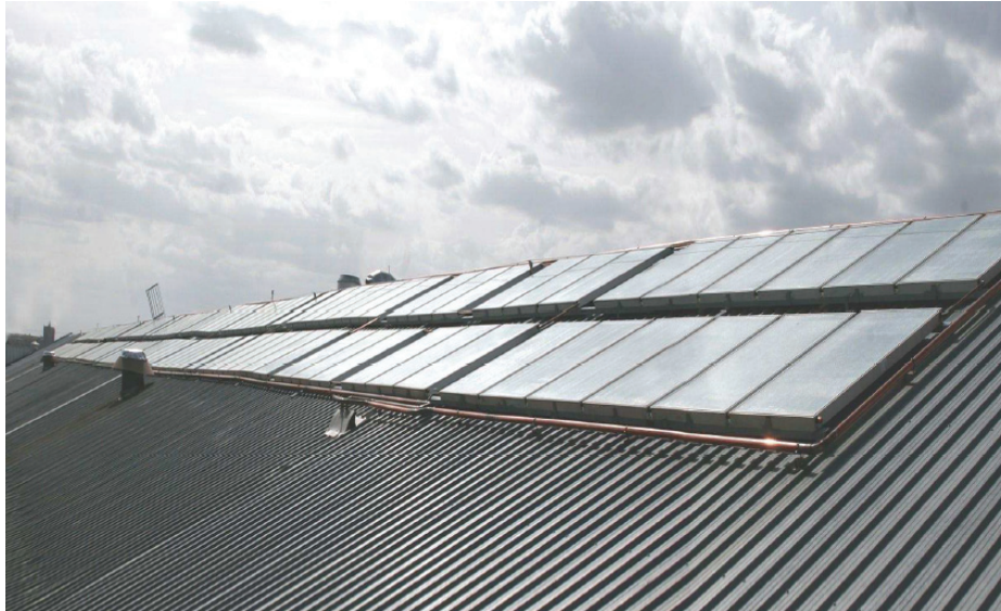
Solar thermal installation in Industry
